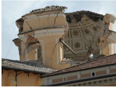
Fig.3. Church of S. Maria del Suffragio, Aquila, Italy. Seismic failure of the dome. [11]
