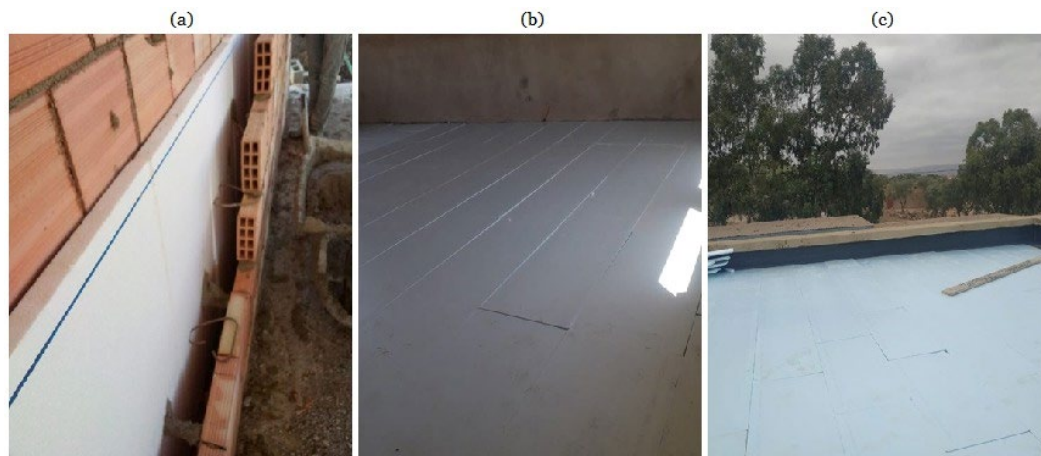
Fig. 6: Installing polystyrene as insulation in the building envelope: (a) external wall, (b) floor on ground, (c) roof.
